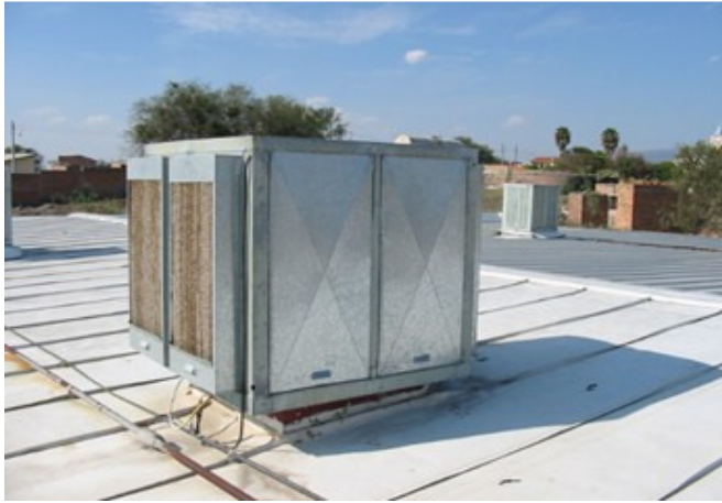
Photo 1: Evaporative cooling Unit on the roof of a hatchery
