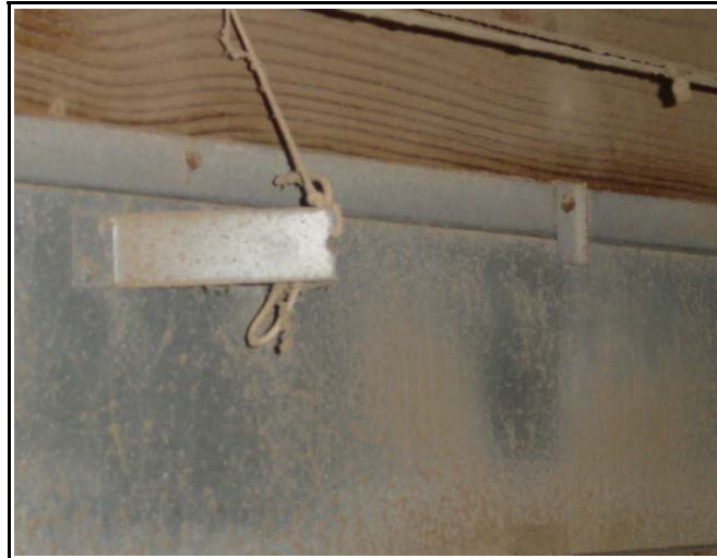
Figure 9. Air inlet latched closed.
