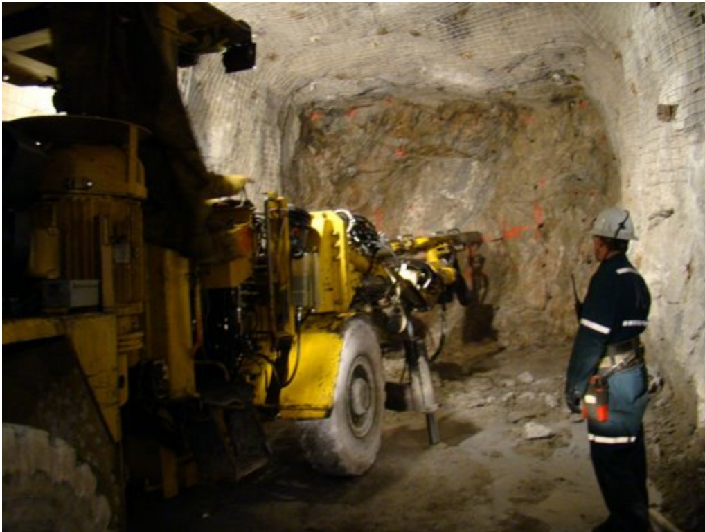
Fig. 4. Mechanized drilling at the Rabbit Lake underground mine. (Photograph by A. Liu, DFO)
