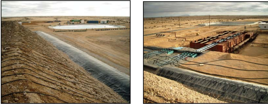
Plate 4.5: Trekkopje mini heap leach pad and storage tanks for the ‘pregnant leach’, during early trial stages of the mine design and construction in 2008 (photo Geological Survey).
