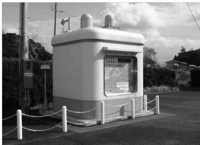
Fig.5 Appearance of monitoring station
